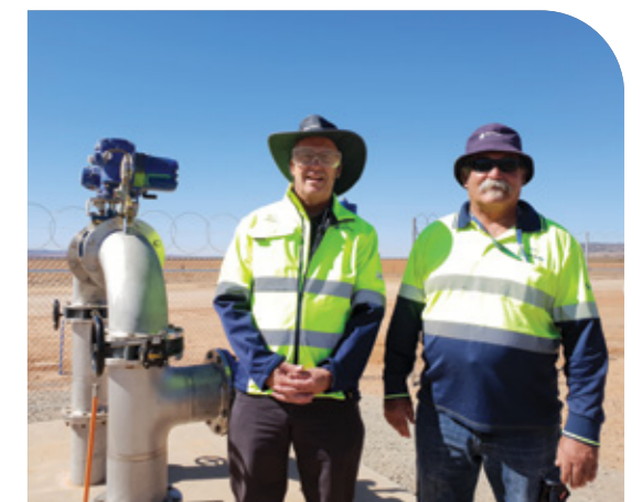
Orroroo pipeline infrastructure
